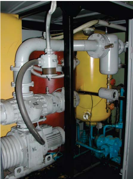
TRANSFORMER OIL DEGASSING UNIT
